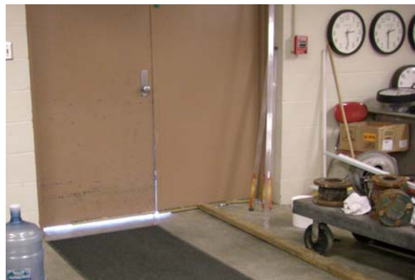
Figure 5. Gaps under doors invite pests into the school building.
