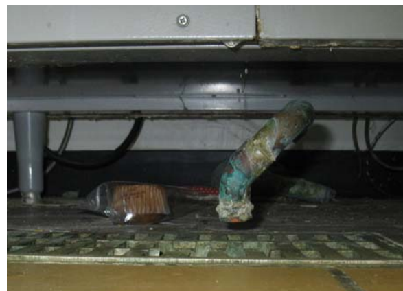
Figure 3. Food and trash found under kitchen equipment attracts pests.
